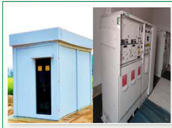
Dedicated RMU Building for each plot for electricity and Optical Fiber Connection
