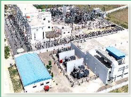
Dedicated 220/33 & 33/11 Electric Sub-Station for uninterrupted high quality power supply
